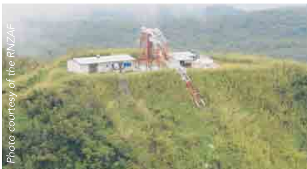
Figure 1: A tower which failed in Tropical Cyclone Tomas in 2010.
